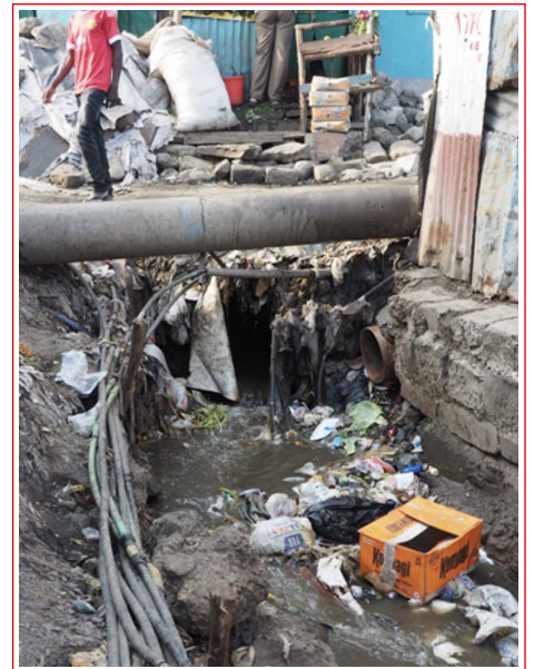
Figure 1. An open sewer and informal water pipes in Mukuru, Nairobi, Kenya.
