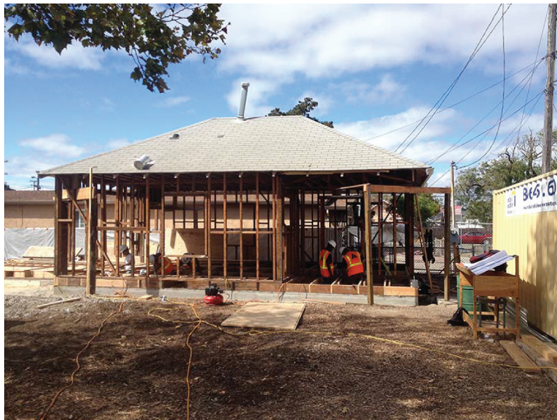
Figure 6. Rebuilding house adjacent to Elm Playlot into an office, kitchen and bathroom (Source: Pogo Park).
